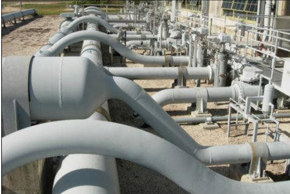
Figure 19. Station suction and discharge piping. Courtesy Pipeline Knowledge & Development.
