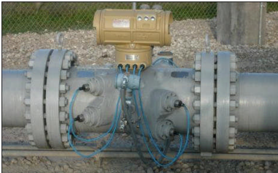
Figure 23. Ultrasonic meter on a pipeline interconnect. Courtesy Pipeline Knowledge & Development.
