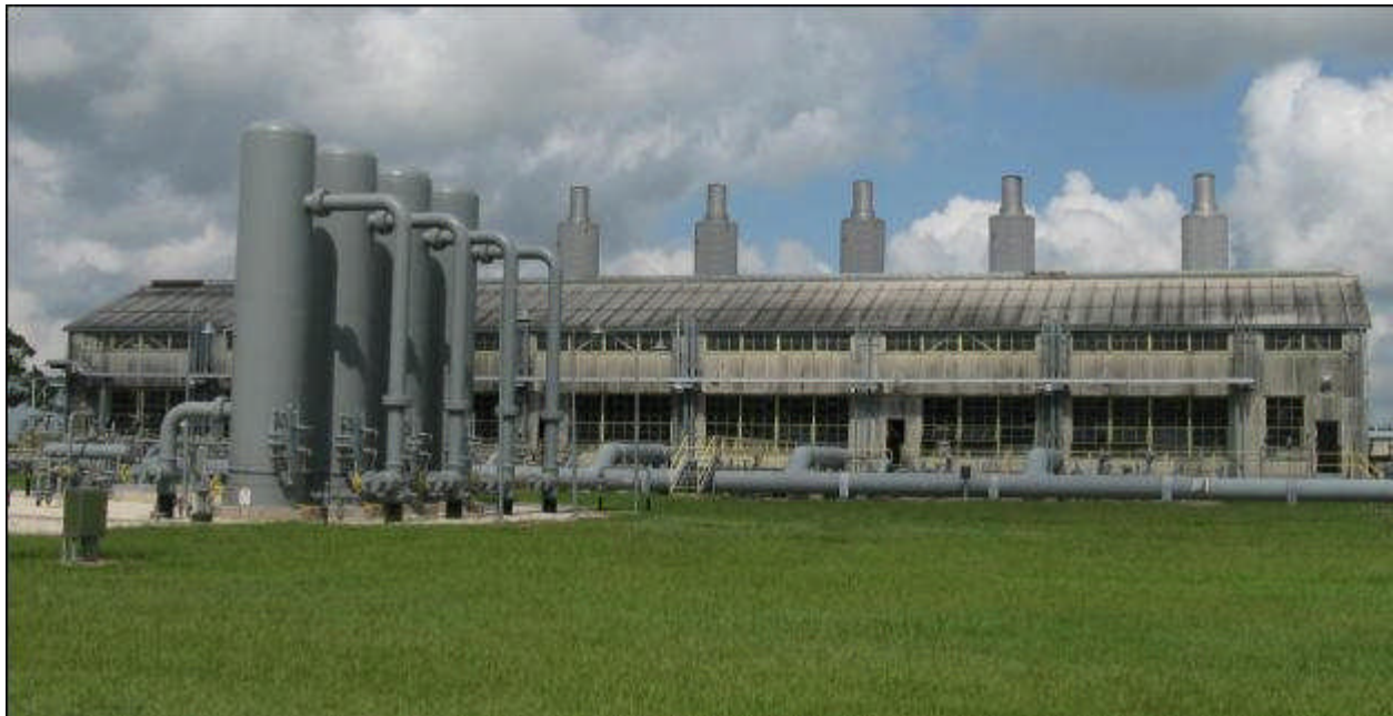
Figure 14. Natural gas compressor station with scrubbers. Courtesy Pipeline Knowledge & Development.
