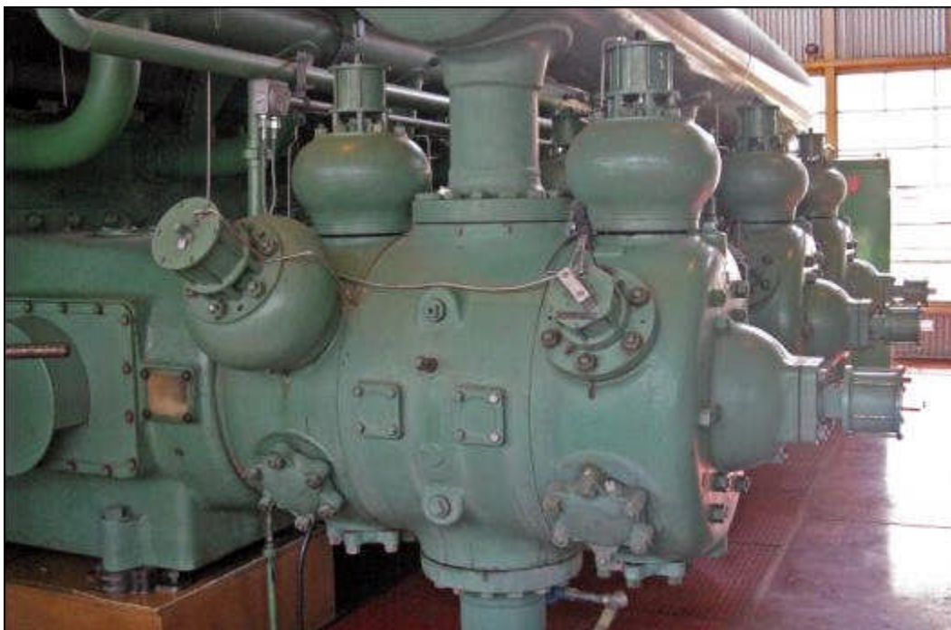
Figure 21. Reciprocating compressor. Courtesy Pipeline Knowledge & Development.
