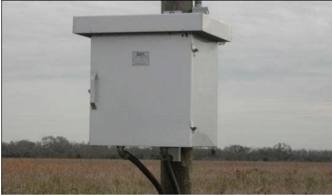
Figure 41. Rectifier. Courtesy Pipeline Knowledge & Development.
