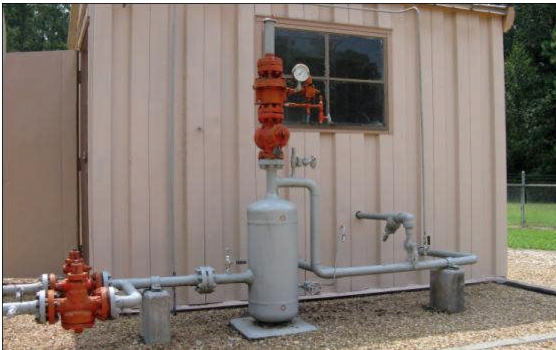
Figure 37 Station Drip. Courtesy Pipeline Knowledge & Development
