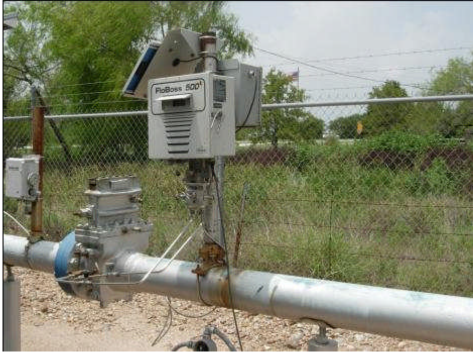
Figure 22. Orifice meter on receipt line. Courtesy Pipeline Knowledge & Development.
