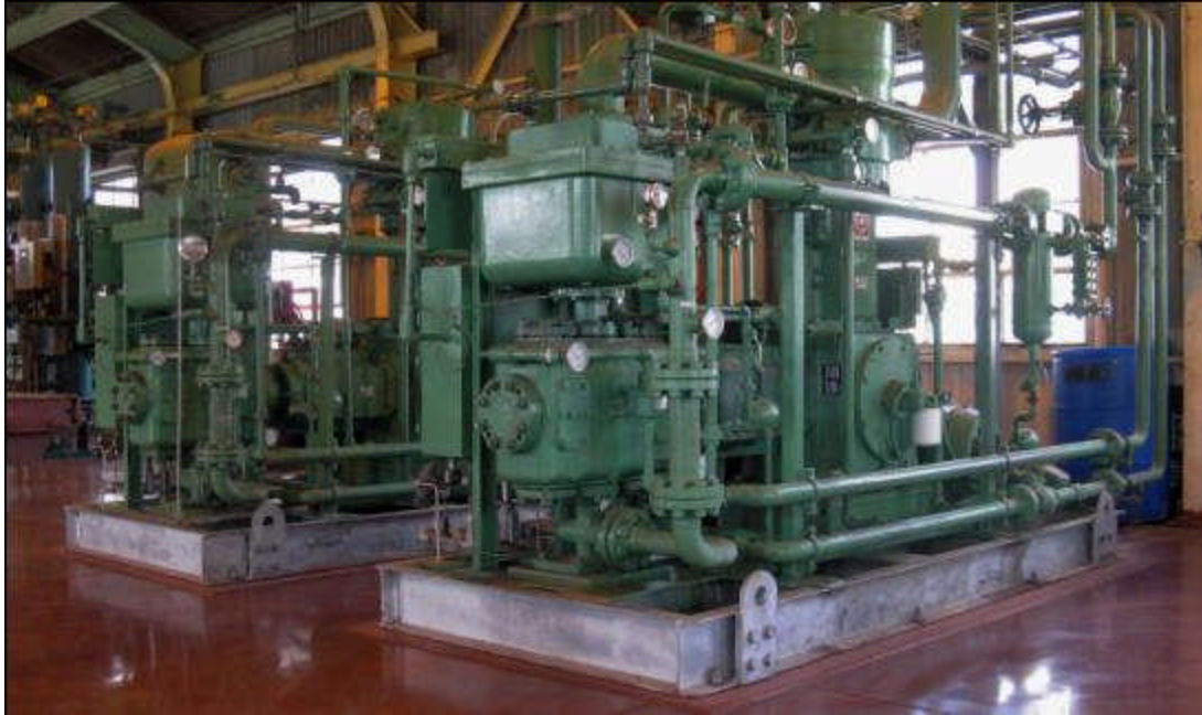
Figure 42. Air compressors in compressor station with engine drivers. Courtesy Pipeline Knowledge & Development.
