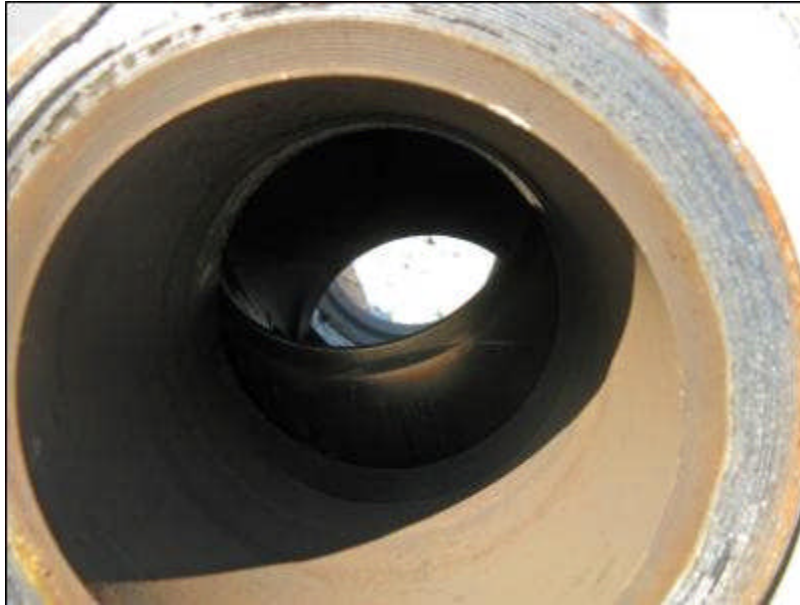
Figure 31. Partially open ball valve. Courtesy Pipeline Knowledge & Development.
