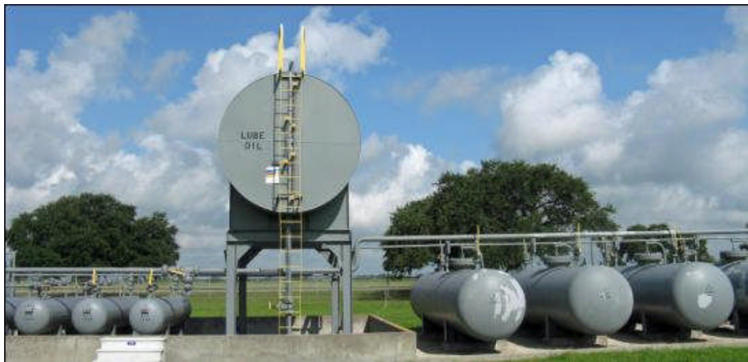
Figure 43. Compressed air storage cylinders. Courtesy Pipeline Knowledge & Development.
