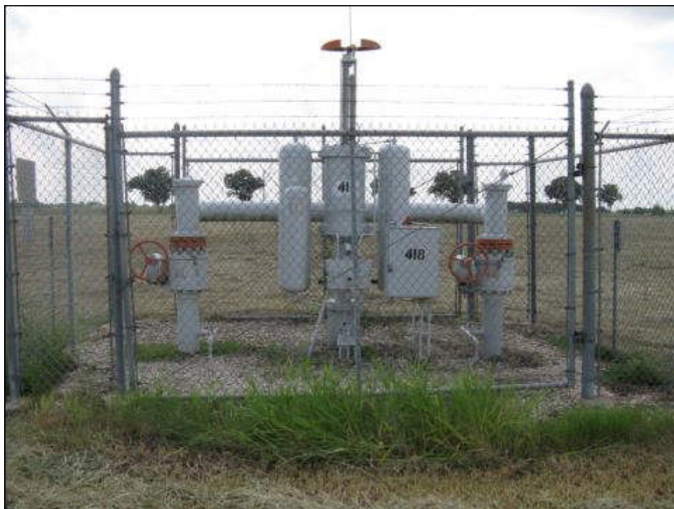
Figure 27. Block valve station. Courtesy Pipeline Knowledge & Development.
