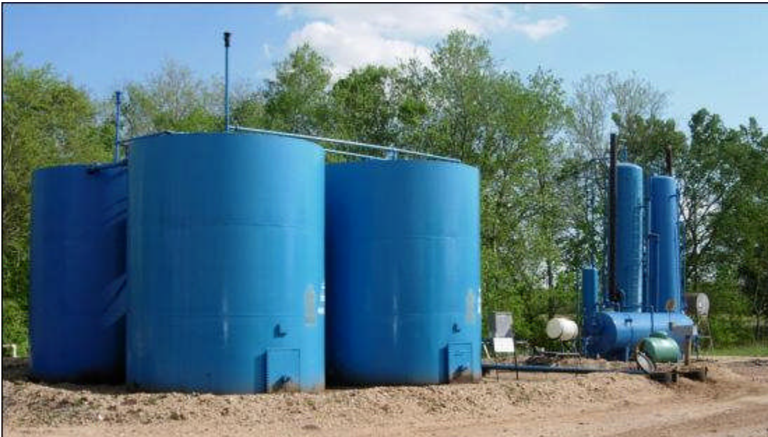
Figure 2. Lease separators and oil tanks. Courtesy Pipeline Knowledge & Development.
