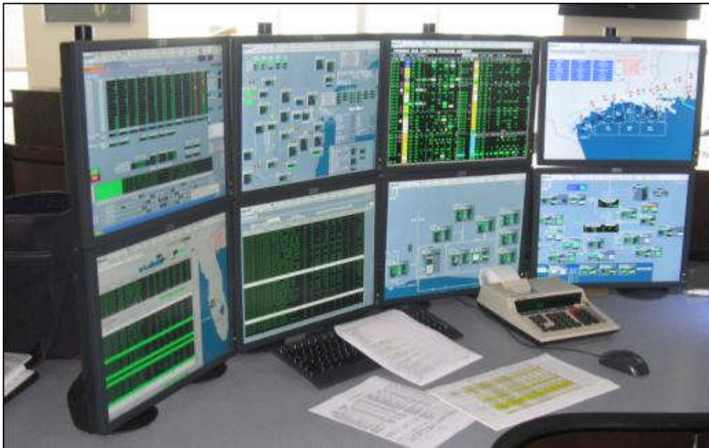
Figure 45. Control room operating console. Courtesy Pipeline Knowledge & Development.
