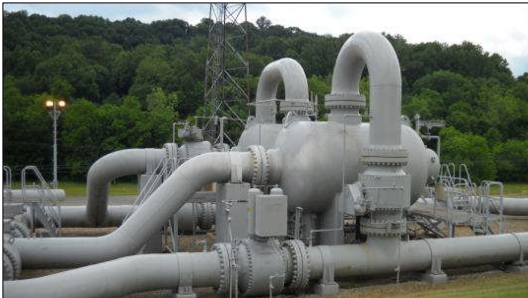
Figure 40. Horizontal Filter Separators.
