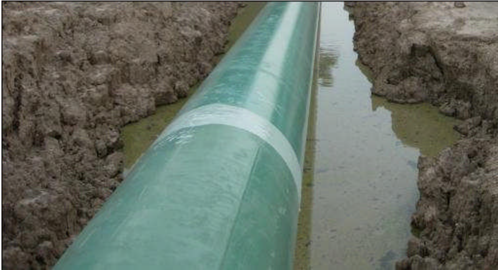
Figure 30. FBE coated pipe with field coating applied to girth weld. Courtesy Pipeline Knowledge & Development.
