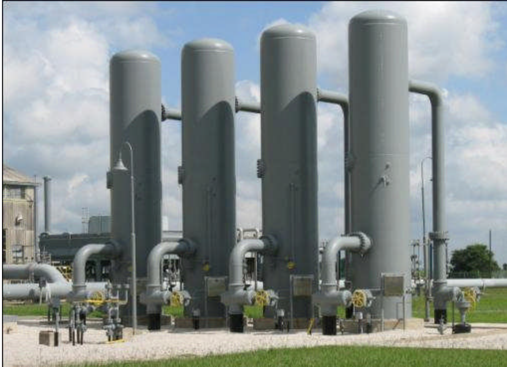
Figure 39. Natural gas scrubbers. Courtesy Pipeline Knowledge & Development.
