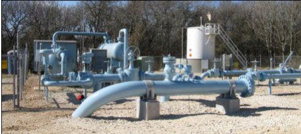
Figure 26. City gate station. Courtesy Pipeline Knowledge & Development.
