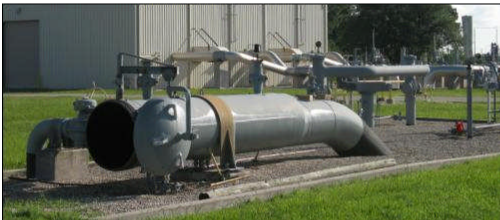
Figure 20. Station piping. Courtesy Pipeline Knowledge & Development.
