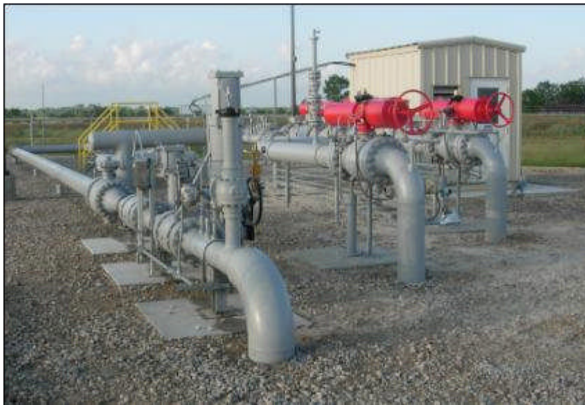
Figure 24. Interconnect station. Courtesy Pipeline Knowledge & Development.
