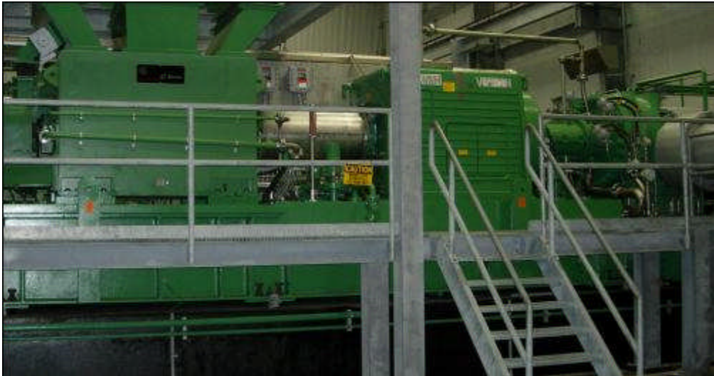
Figure 17. Centrifugal compressor driven by an electric motor through a variable speed drive. . Courtesy Pipeline Knowledge & Development.
