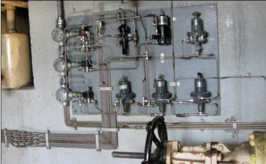
Figure 44. Instrument air control manifold. Courtesy Pipeline Knowledge & Development.
